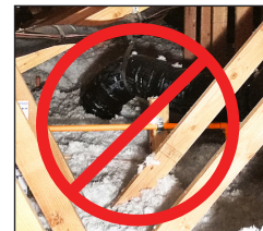
INCORRECT (Exposed piping)
