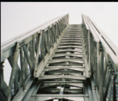
No "K" bracing to impede the footpath.
