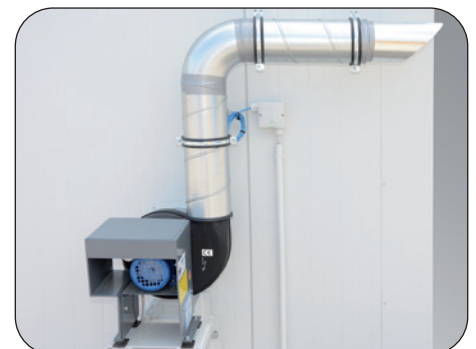
Ex-proof exhaust fan incl. exhaust air monitoring
