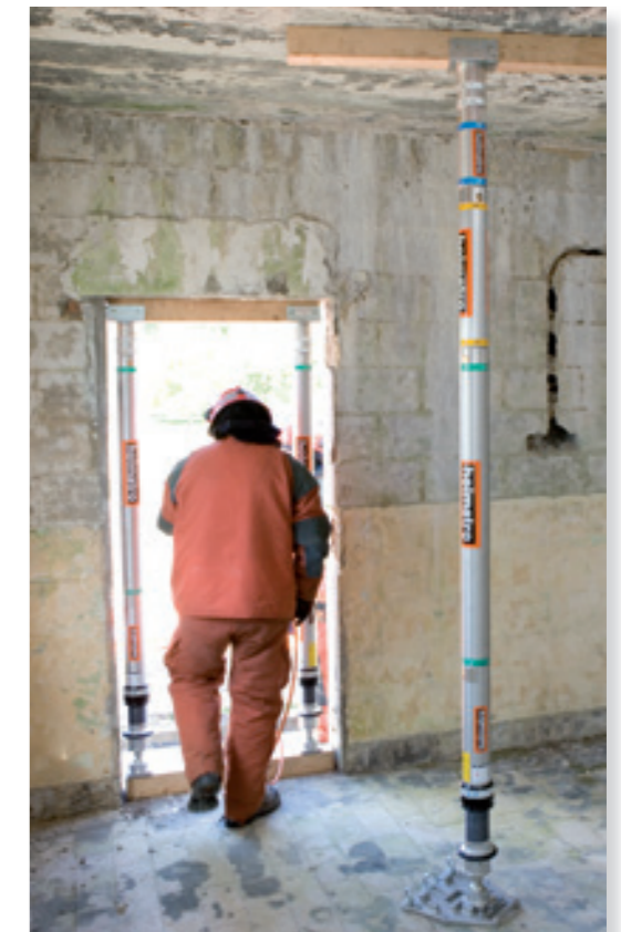
Shores combined with timber to protect the access and exit route of a collapsed building.
