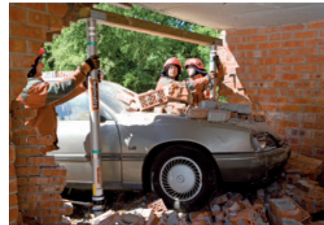
Positioning two shores with beam support heads and a beam, to stabilize a building. The hydraulic Locknut struts will be carefully extended by means of a hand pump.
