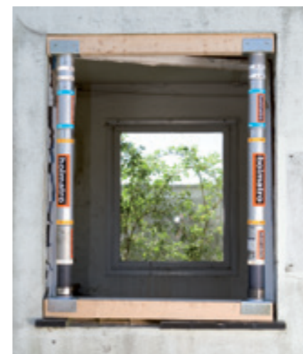
Manual struts with extensions, beam support heads and timber to stabilize a window.
